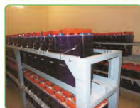
Kingdom of Cambodia's power station
